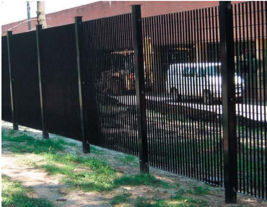
New fencing at the Arlington Water Pollution Control Plant is just one of several ongoing upgrades to the facility. Portions of the fence along S. 31st St. have already been installed.
