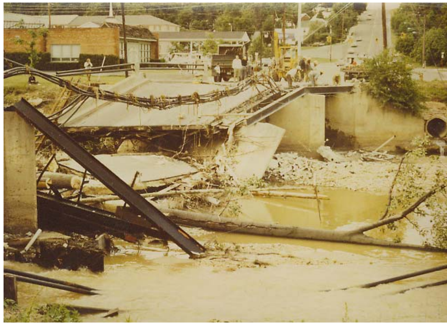
Figure 4 Collapse of the Walter Reed Bridge in Arlington County – Just Upstream of the USGS Gaging Station. Flooding on June 22, 1972 was due to the remnants of Hurricane Agnes.
